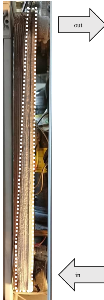
Figure 12: Ice formation on evaporator at B0/W35, 60Hz and SH10K, system 1
